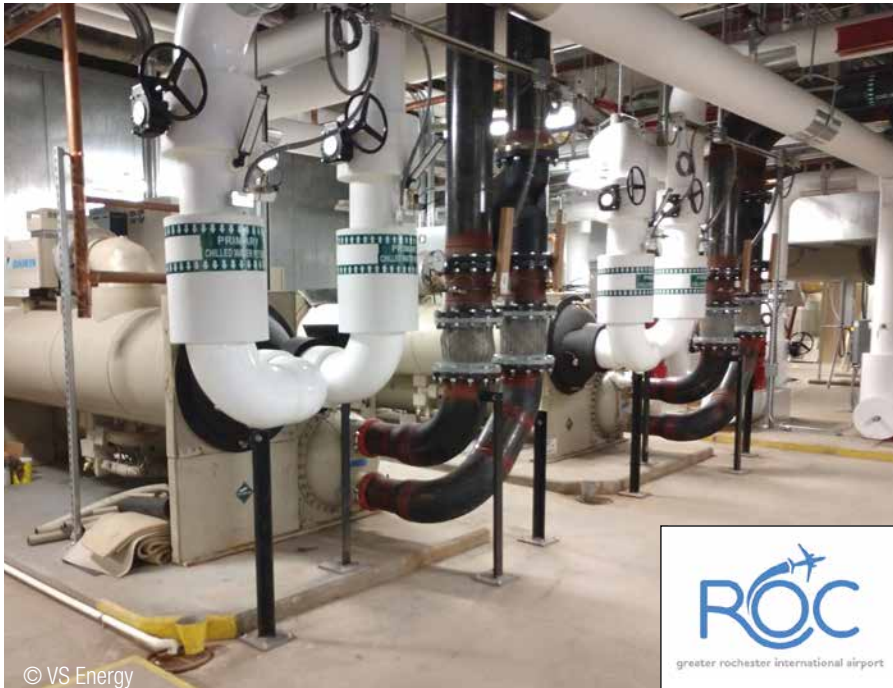
© VS Energy Daikin Magnetic Bearing Variable Speed Drive Chillers
