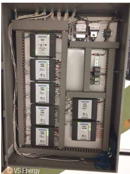
© VS Energy Alerton AAC - Advanced Application Controller with expansion modules for the central chilled water plant
